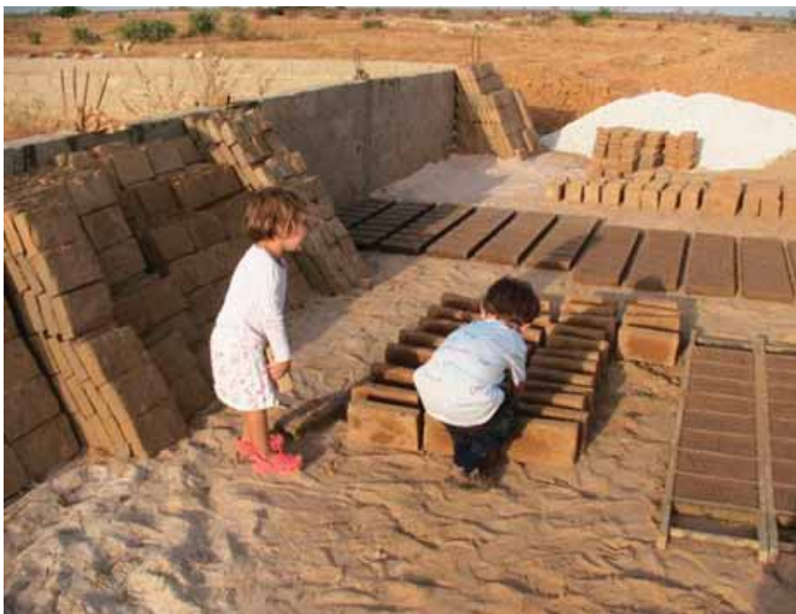
The author’s children were an integral part of the process of building the family’s earth house. Here, at ages three and four, they help make the bricks that will be used for doorways and arches.
